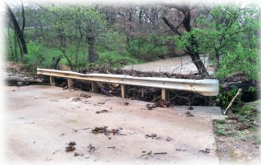
Stormwater flooding in Benton County
