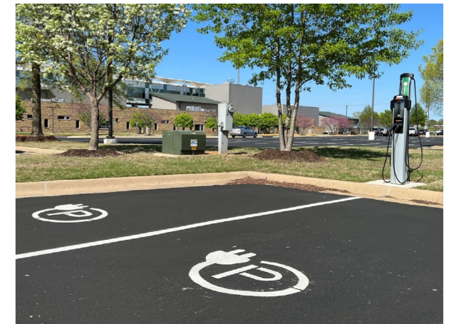
ARVEST Baseball Park in Springdale, EV charging stations
