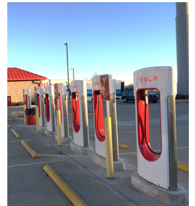
Workman's Center in Lowell EV charging stations
